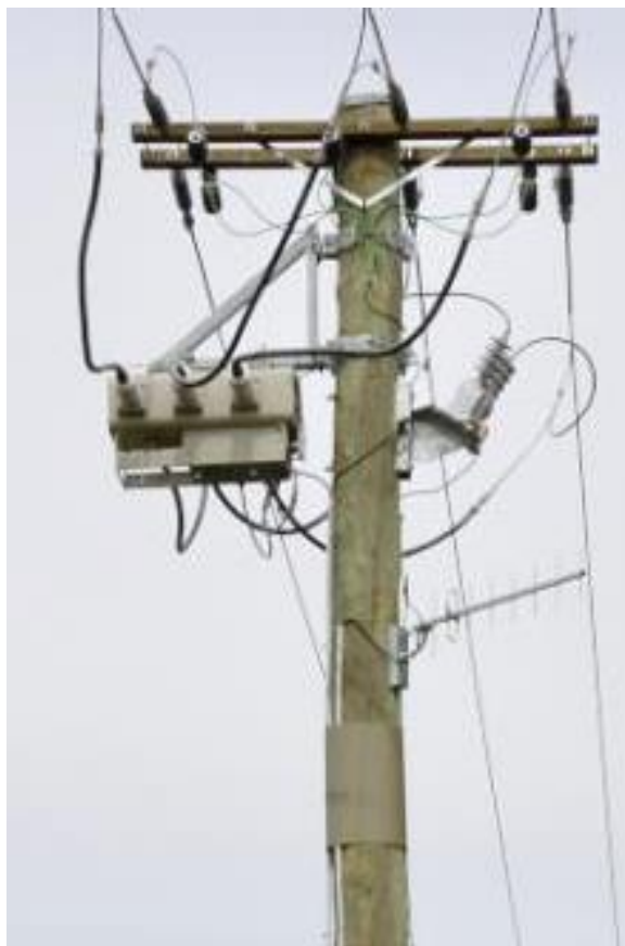
Pole Mounted Vacuum Switch – with communication antenna and power supply VT
