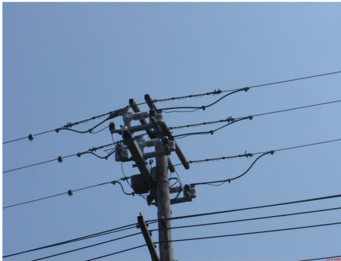
S&C Scada Mate Switch A1 Switch Side
